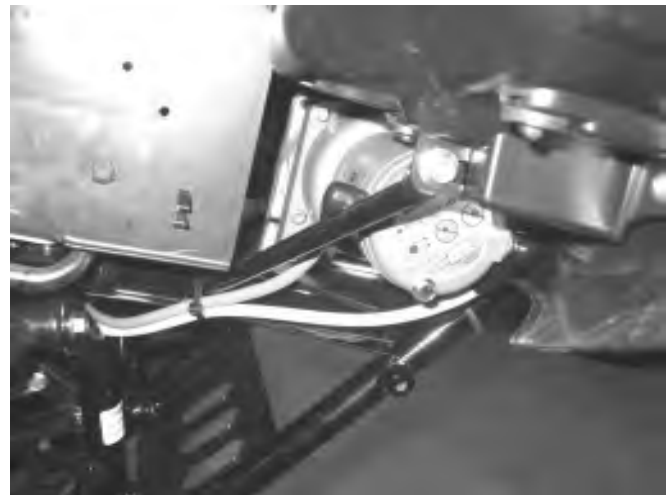
Figure 28 Electrical Cable Routing - Contactor to Winch
